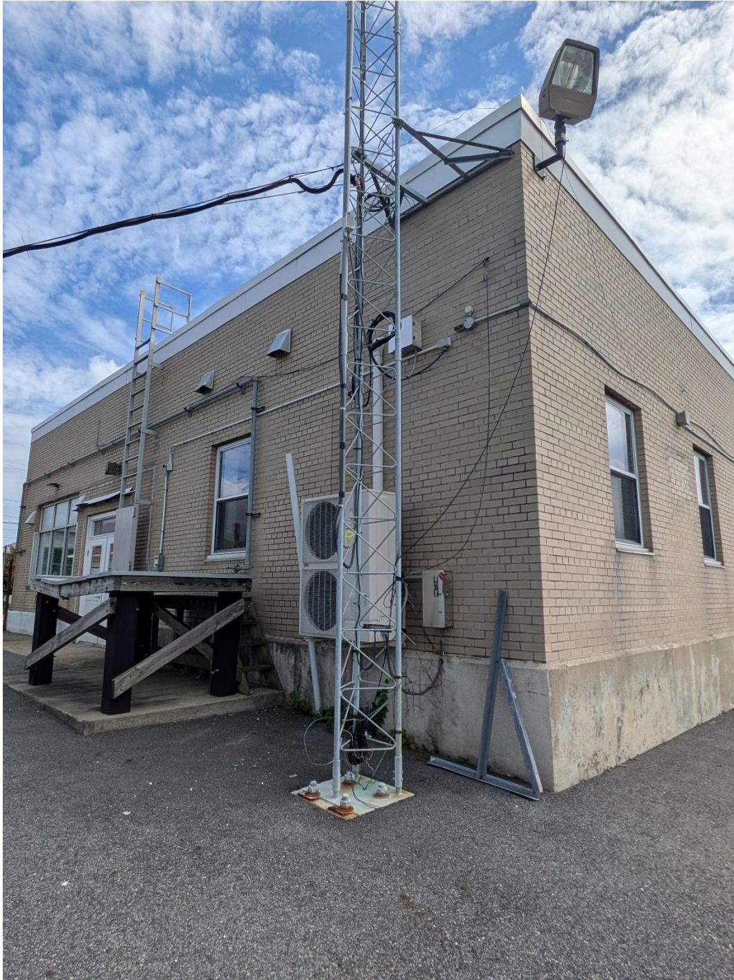
Rohn Tower at the Town's Marine Laboratory and Biological Field Station in Point Lookout.
